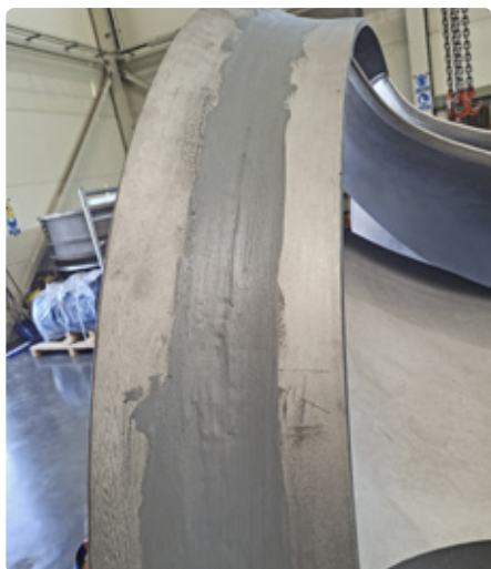
Fig. 3. Reprofiting of rotor surfaces – filling of pits and irregularities with Belzona®1111 composite
