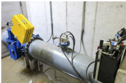
Fig. 5. An example of throttle installation activated by an over speed sensor
