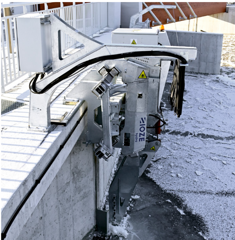
Photo 6. Horizontal trash rack cleaner supporting the operation of the facility
