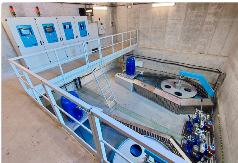
Photo 4. Interior of the SHP with two hydro units and control platform
