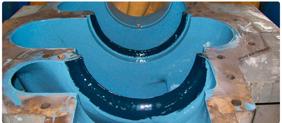
Photo 6. Pump body after filling the pitting with the Belzona®1311 composite, rehabilitation by means of the Belzona®1341 coating and applying Belzona protective coating
