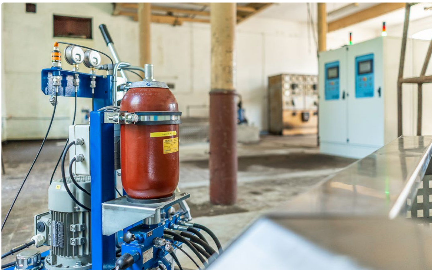
Photo. A hydraulic unit, new control cabinets and historical elements of the mill equipment in the background
