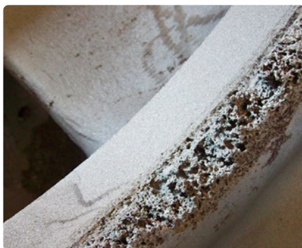
Photo 5. Cavitation pitting in the surface layer of the pump body
