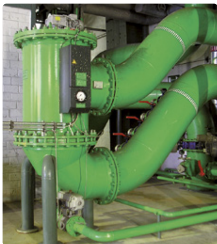
Photo 1. Process water filter, RF3-5 type, Q = 1500-2450 m 3 /hour
