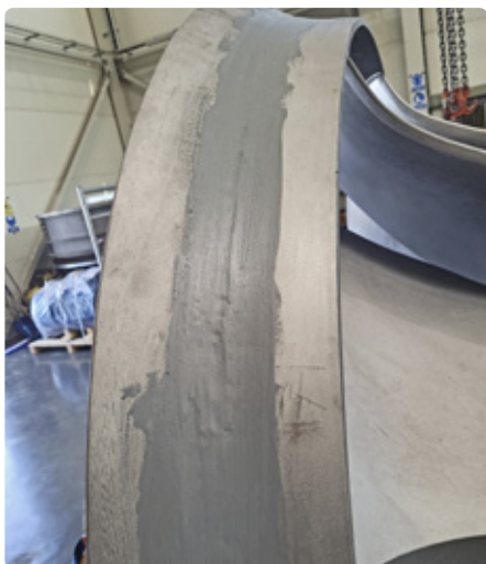
Photo 3. Reprofiting of rotor surfaces – filling of pits and irregularities with Belzona®1111 composite
